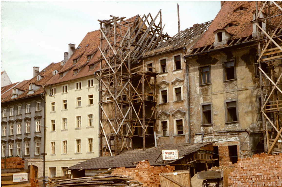
Renovation work begins in the western Bohemian town of Cheb (German: Eger) after more than a decade of decay post-expulsion. The signs in the bottom picture advise that a drugstore behind the construction site is open, with cosmetics and photographic film for sale.
